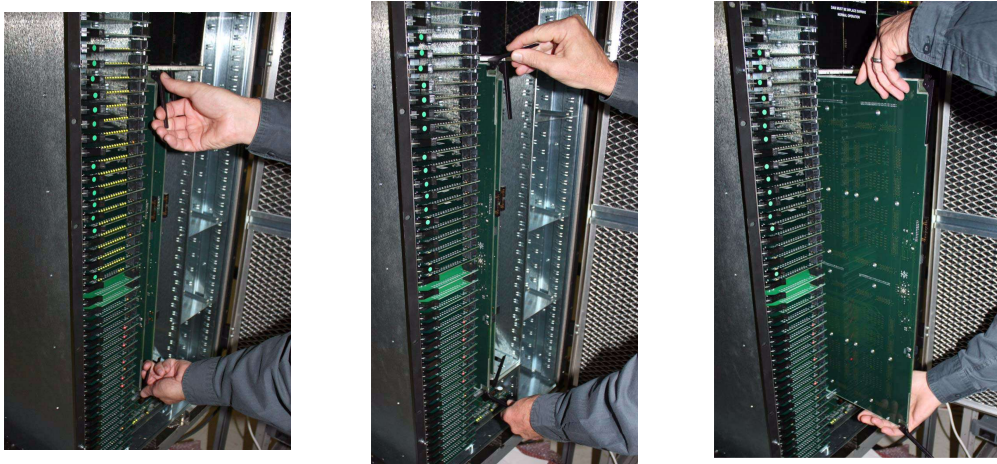
FIGURE 3-11. Crosspoint Board Removal
